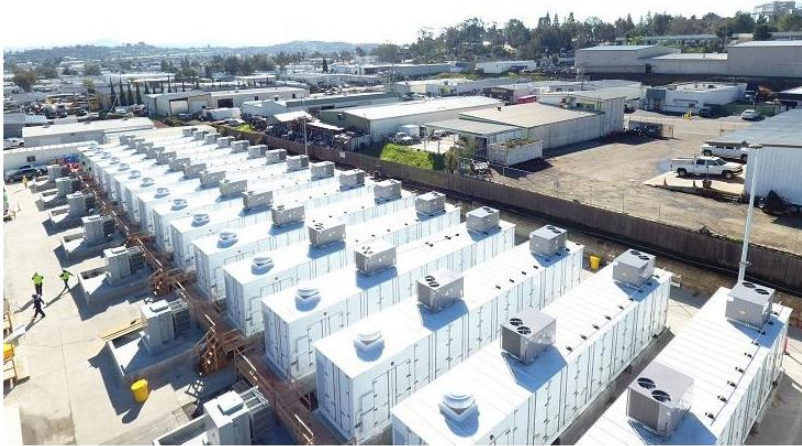
Photo courtesy of San Diego Gas and Electric Co.
